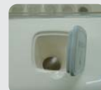
Water supplyment for humidification
