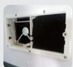
Centralized Heating & Humidification unit
